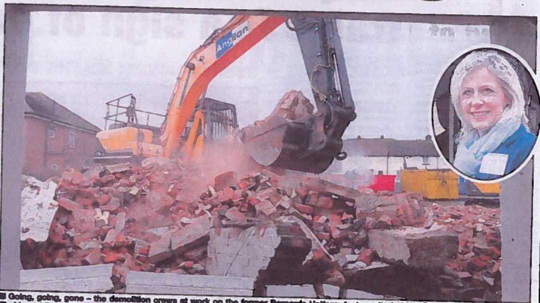
Going, going, gone - the demolition crews at work on the former Bernards Uniform factory site in Main Road, Harwich. Inset: Sara Thakkar of Colne Housing Society, which is building 27 affordable homes on the site. Pictures: STEVE BRADING 0011477
